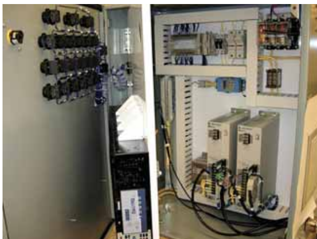
Interior components of Remote Valve Actuator Controller
